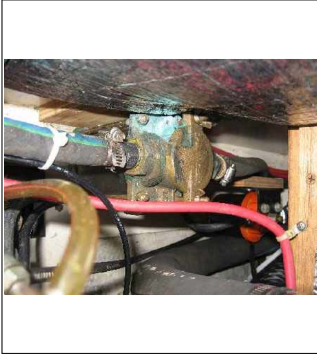
Finding C.5 Corrosion on Engine Raw Water Filter
